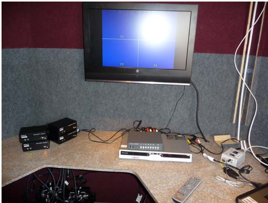
Figure 19. Quad Switcher, DVR, Wall Monitor, and Commbox
